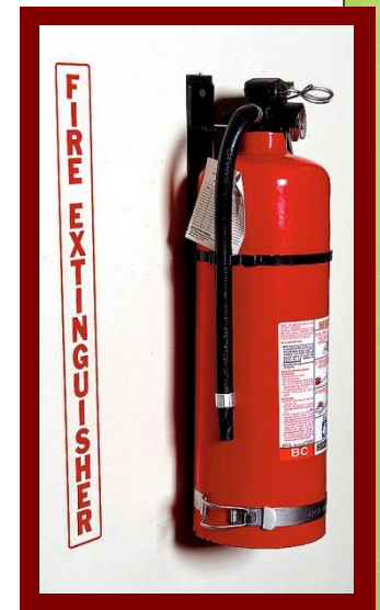
Fire extinguishing equipment
