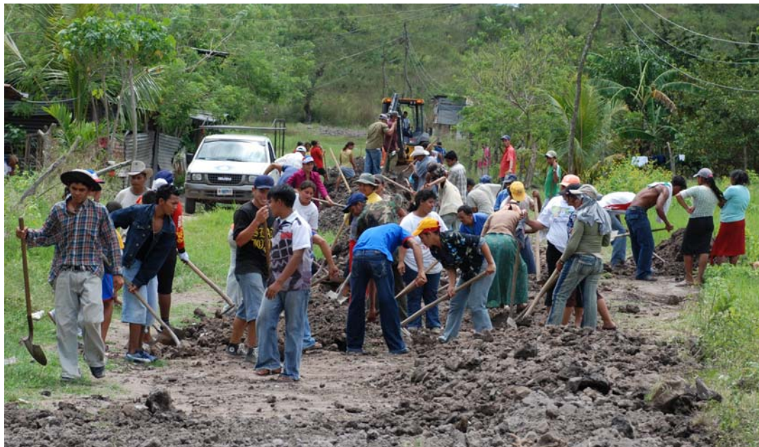
Figure 5.2: Approximately 50 local people of Colinas de Suiza are working to lay pipe for their water distribution system.
